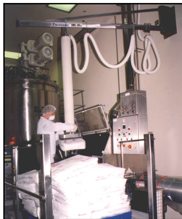
Wall mounted swing jib arrangement and vacuum tube lifter handling sacks from a pallet into a sack tip booth.
